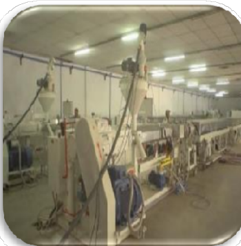
Pipe Extrusion Facility
