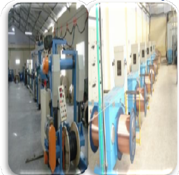
Cable & Wire Facility
